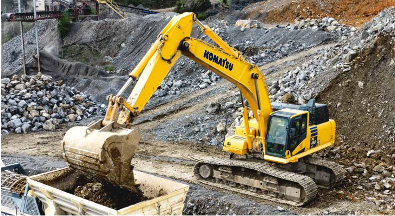
An operator uses a Komatsu PC490LC-11 excavator to load a crusher with limestone.
