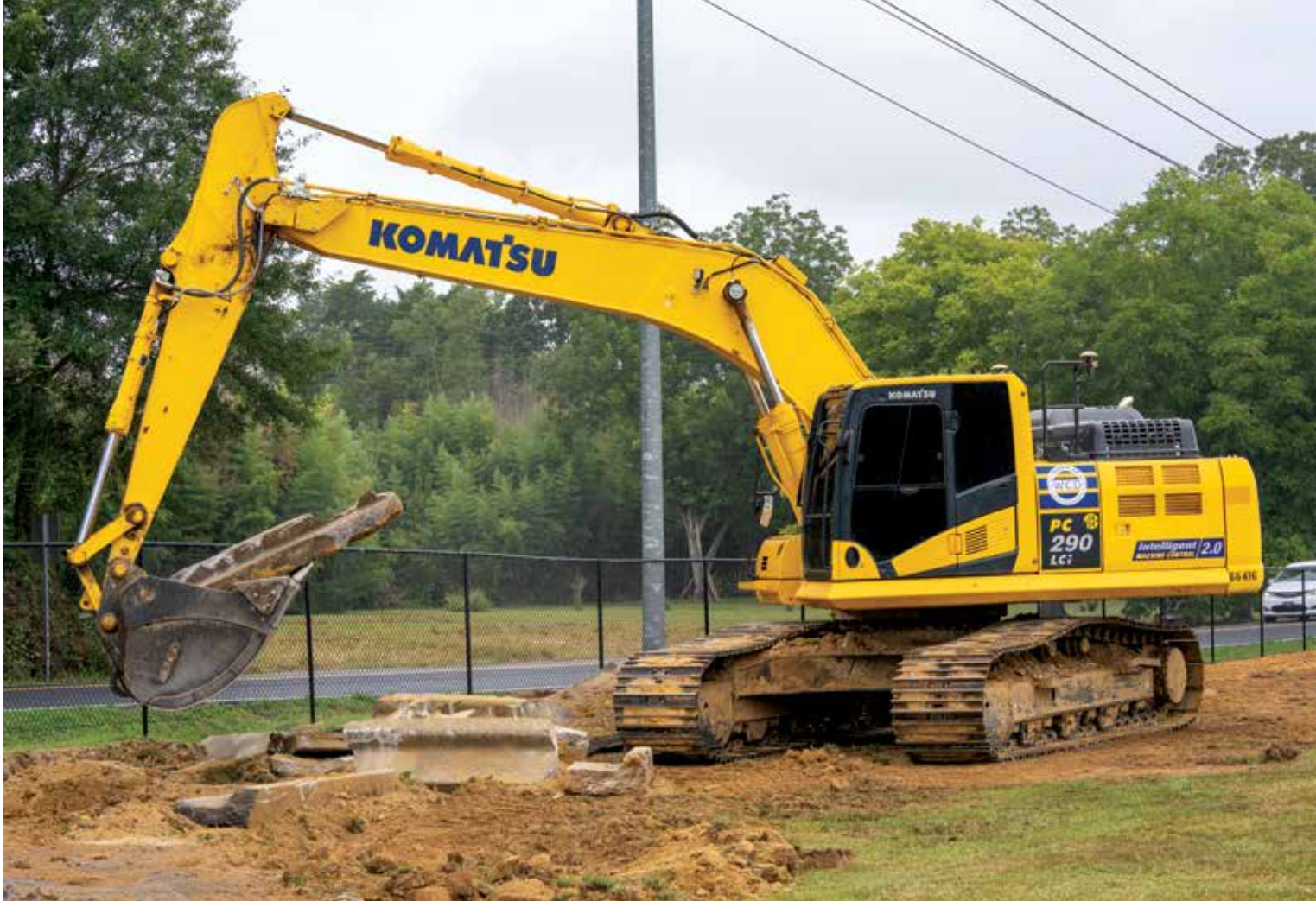
Removing asphalt and concrete curbing is no problem for midsize excavators like the Komatsu PC290LCi-11 IMC model.
